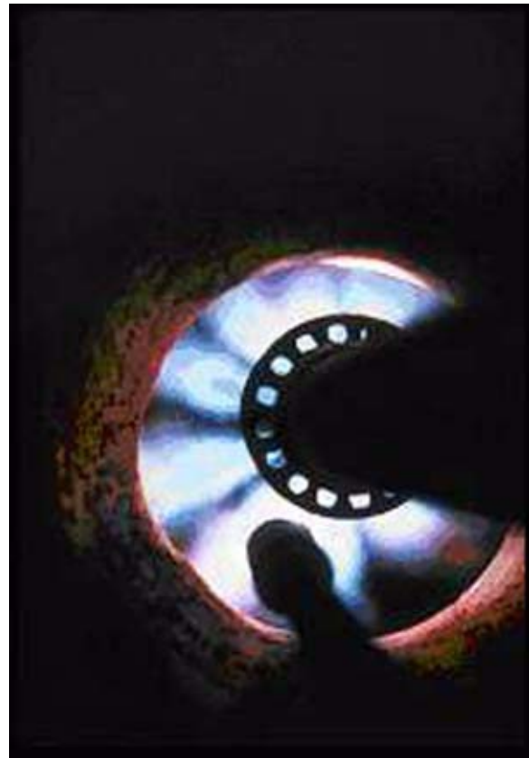
Figure 38—Improper Burner Tile Installation Leads to Poor Flame Pattern
