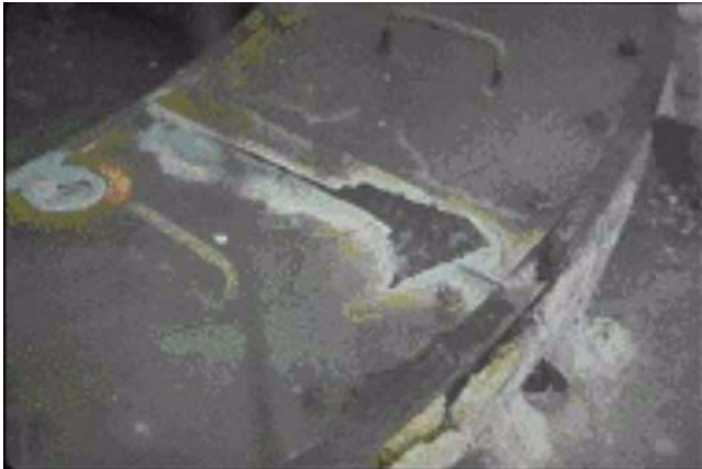
Figure 17—Dew Point Corrosion from Flue Gas Corrosion on Radiant Section Header Box
