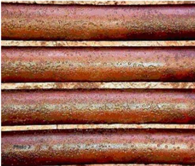
Figure 11—General Metal Loss and Pitting of Tubes After Exposure to Moisture and Corrosive Deposits During Idle Periods
